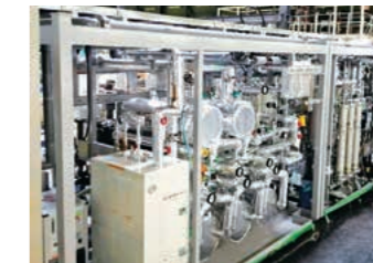
NMP refining and recycling system
