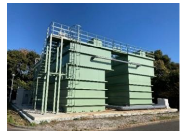
Full scale GFT at Tokyo 8MGD demo
