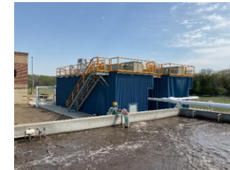
Granule forming tank currently in operation in the United States
