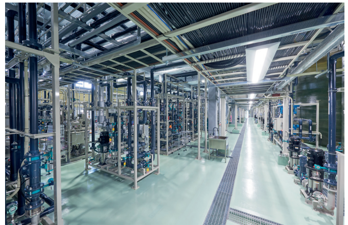
Next generation UPW system at R&D center
